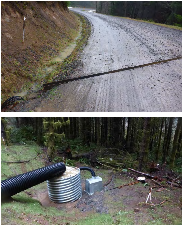
Figure 3.4 The upper figure shows the road surface routing water to the ditch and the collection trough. Water and sediment then are routed through a culvert pipe to the sediment tub. The lower figure shows the platform with the sediment tub collecting road sediment, the tipping bucket measuring discharge and the suspended sediment tank (SST) sampling the fine sediment that is not settled in the tub.
